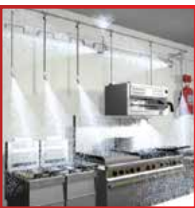
Kitchen Hood Fire Suppression
