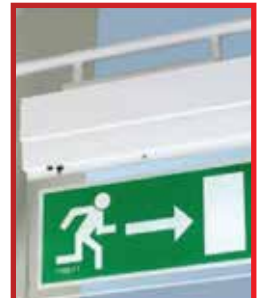
Fire Exit Signs
