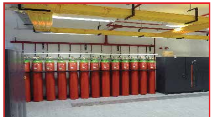
Fire Suppression Systems
